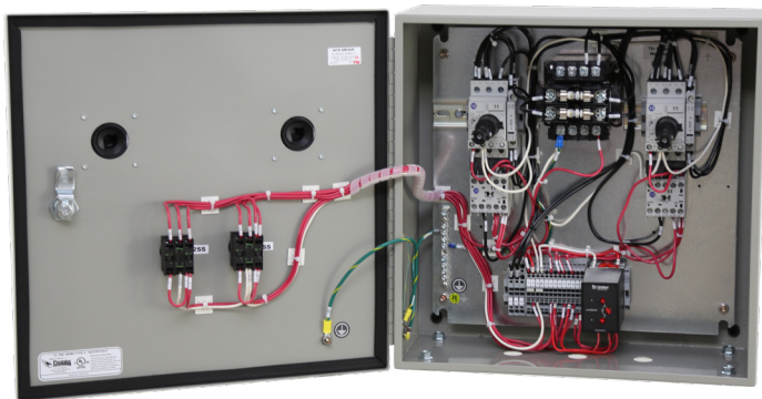
Inside view of control panel
