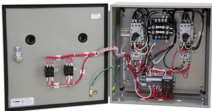
Inside view of control panel
